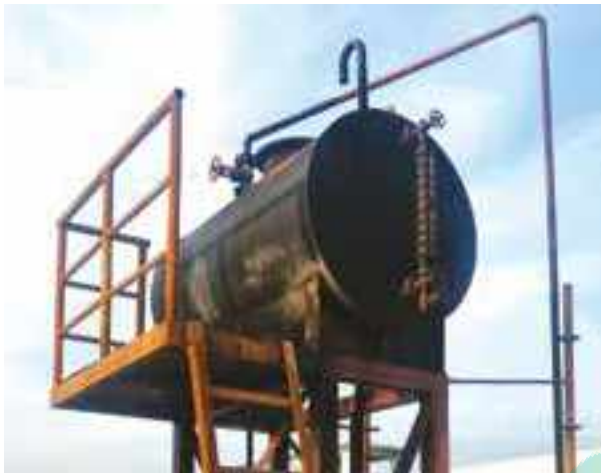
Damaged expansion tank
