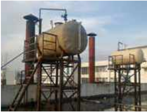
These tanks are unharmed and no fire hazard happened while oil spilled out.
