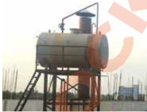
Oil stain marks are visible which is quite normal.
