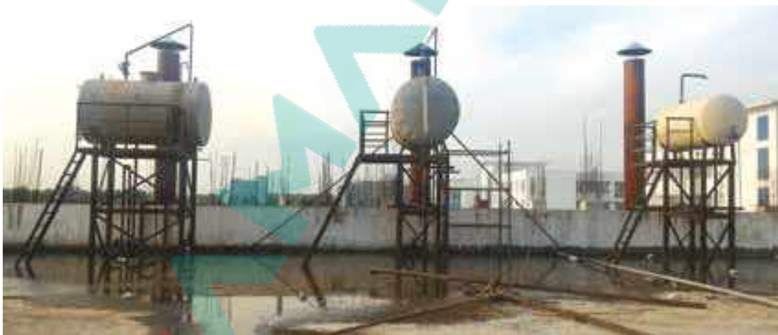
Three more expansion tanks placed separately together.
